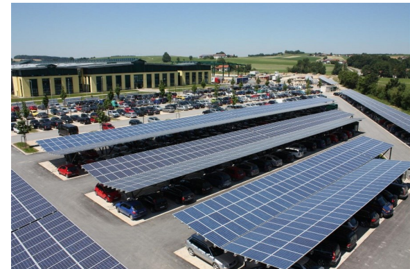
Solar Panel Carports
